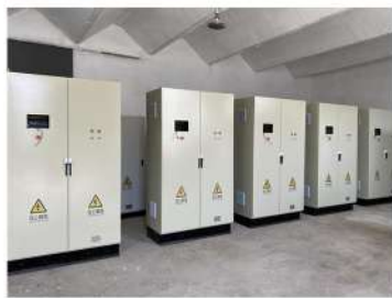
Energy storage system
