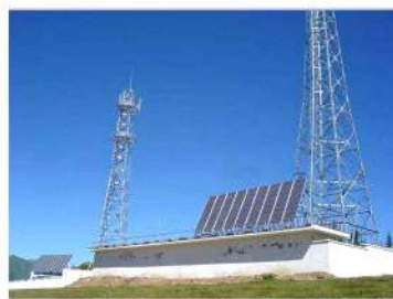
Communication base station, etc.
